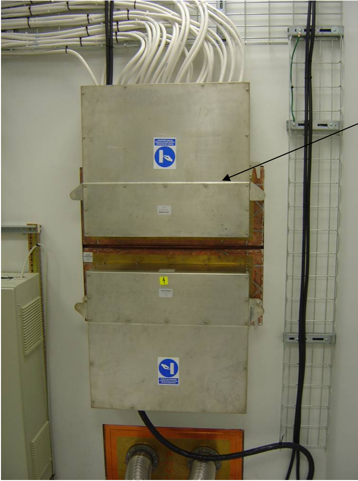
Figure 1 7T Gradient lead filter box (upper unit), RF feedthrough.
