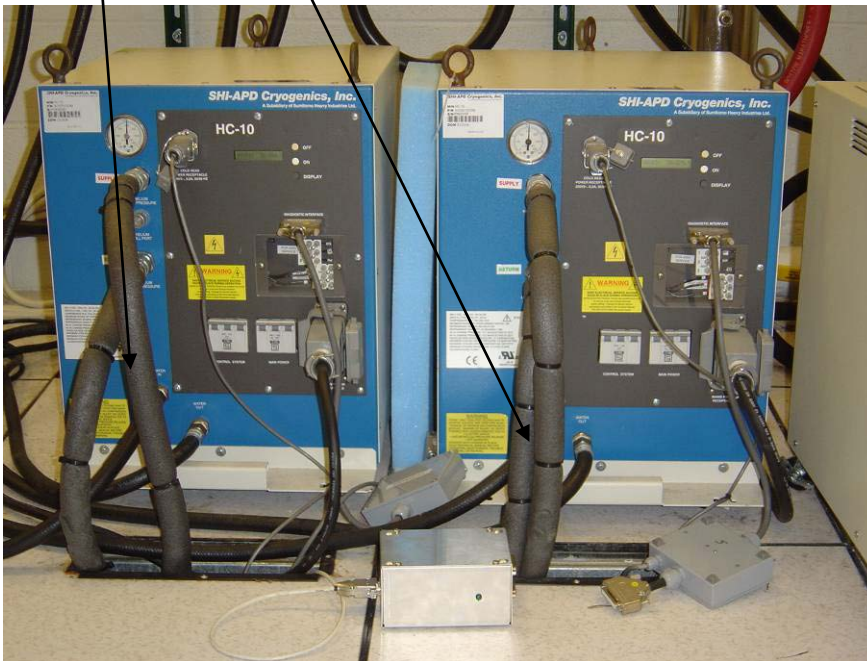
Figure 4 7T Magnet refrigeration units.
