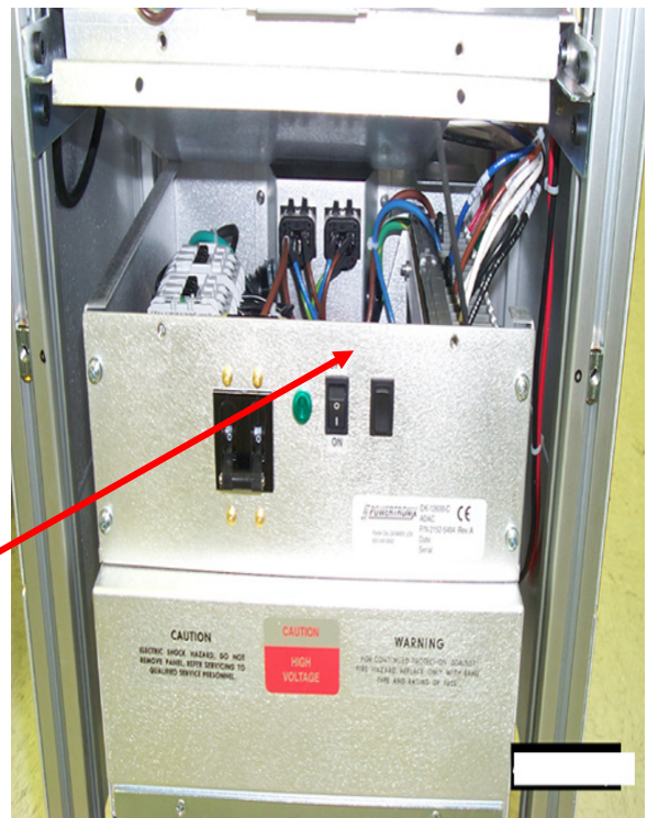
Figure 6 PDU (Inside Power Tower)
